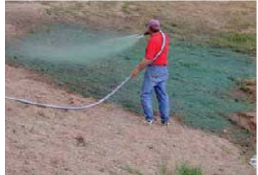
Hydrodraulic soil stabilizers promote the rapid growth of vegetation and prevent erosion.
