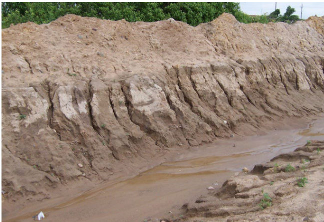
Subsoil erosion at a construction site.
